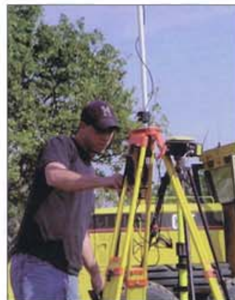
Using GPS+™ and Millimeter GPS™ stakeless grade control systems, Bill Miller says his crew's productivity has doubled. They can bring the initial cut to within final grade tolerances on the first pass.
